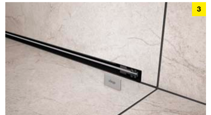
3 After tiling and grouting, the standing grate and cover panel are mounted.
